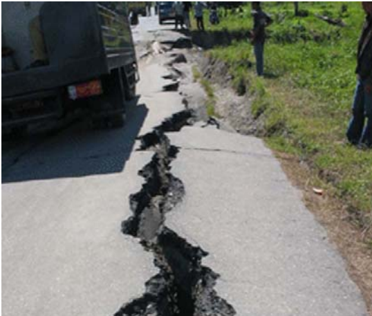
Caption: Cracked road caused by earthquake in Jambi
