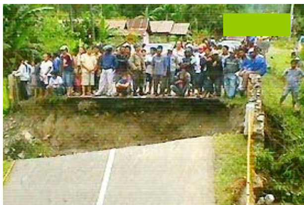
Caption: The broken bridge of Botusuya has cut off the transportation totally. Source: Liputan 6, SCTV
