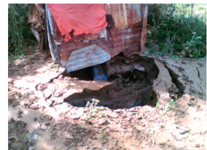
Damaged latrines in Burhakaba
