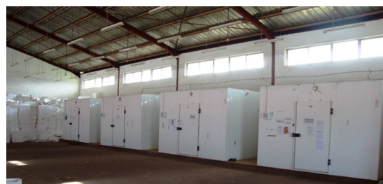
Walk In Cold Rooms at a zonal store. Credit: Souleymane Kone/WHO
