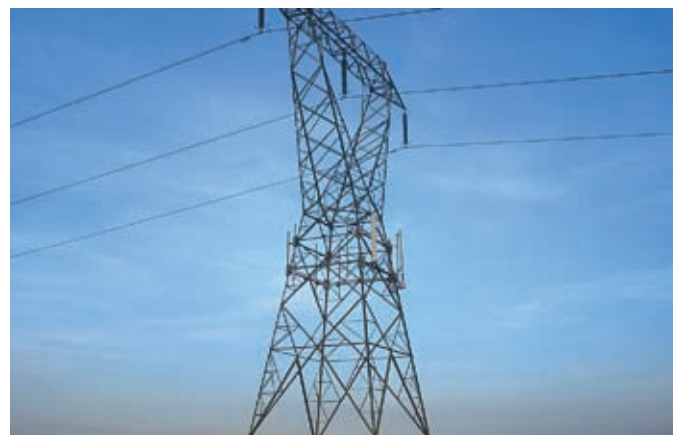
Figure 4.2 Power lines: an important source of ELF fields
