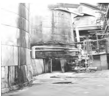
Figure 23.1. Leakages at a production plant
